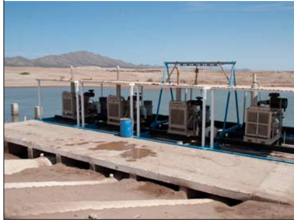
PHOTO 26 Seawater inlet pumps
