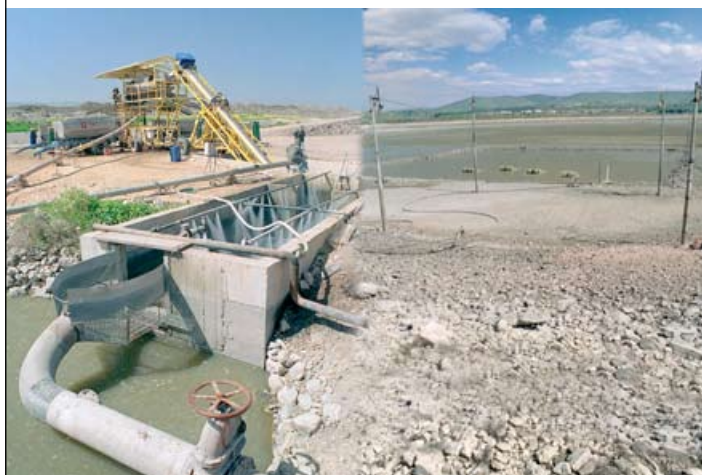
FIGURE 6 A composite picture showing technology for harvesting fish from reservoirs. Top right – drained reservoir with lift-net poles; bottom – draining pipe coming from the reservoir into an external concrete harvesting pit; top left – portable sorting table and “Archimedes screw” fish lift
