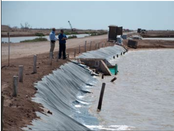
PHOTO 27 Bottom PVC lining in an earthen pond
